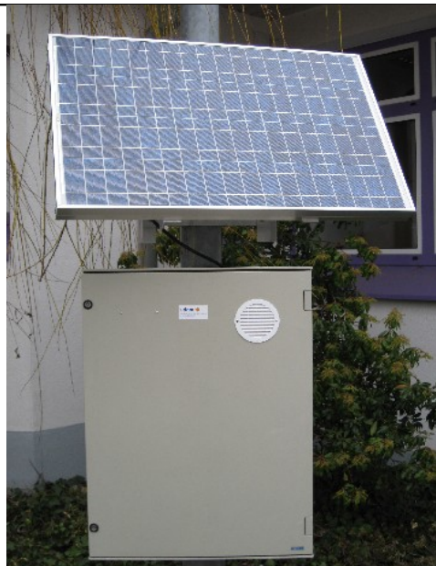
OUTDOOR-CABINET-GFP with Photovoltaic
